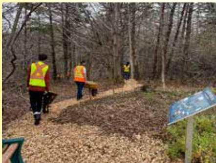
O2 students applying wood chips as trail cover at Van Tassel Lake Trail.
